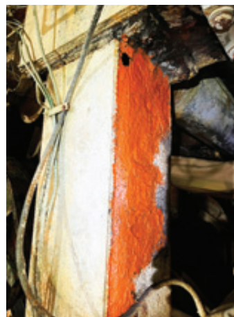
Press post with plate corroded through
