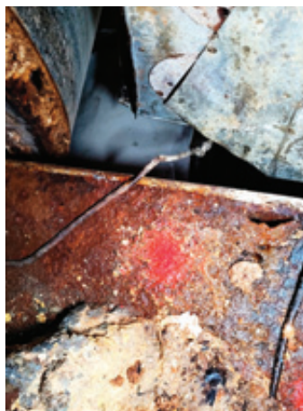
Top of Yankee beam corroded through with side plate evident
